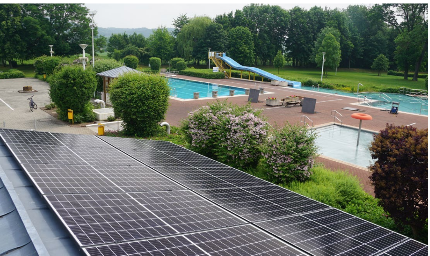
Photo 15: Photovoltaic system on the roofs of the buildings of the leisure and recreation baths © Stadt Bad Köstritz
